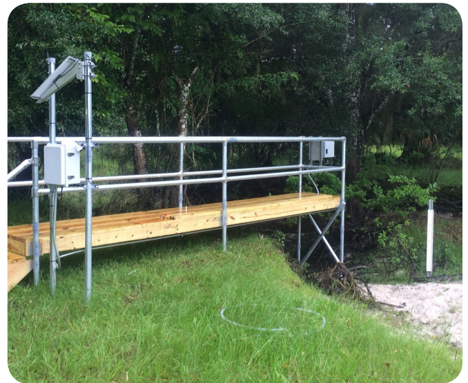
Stormwater monitoring site containing YSI Radar, Data Logger, and Solar Panel. Greenville, South Carolina
