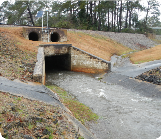
Stormwater monitoring site containing SonTek-IQ®, YSI Sonde, Rain Gauge, Portable water sampler, Customer Data Logger, and Solar Panel. Havelock, North Carolina
