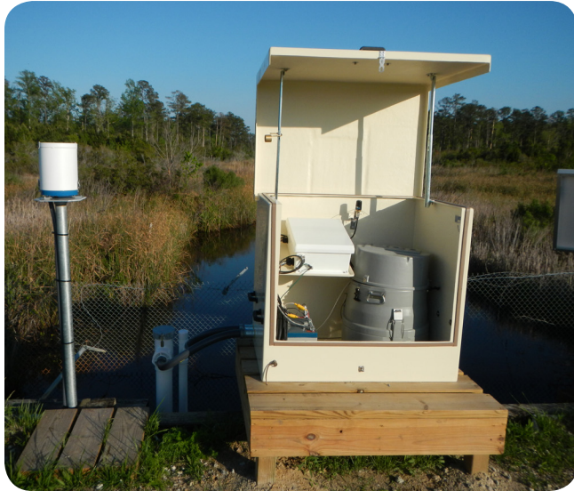
Portable fiberglass clamshell monitoring system containing SonTek-IQ®, YSI Sonde, Rain Gauge, Portable water sampler, Customer Data Logger, and Solar Panel. Havelock, North Carolina
